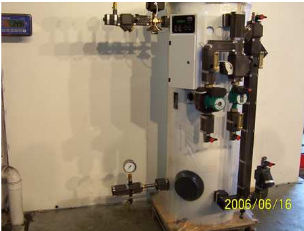
Heat transfer system consisting of a buffer tank, pump, regulator, and heat flow meter.
